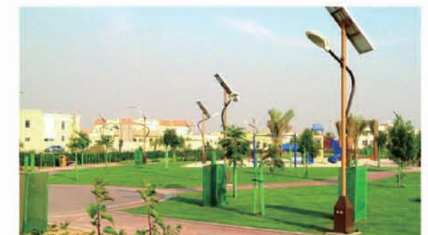
A solar street lighting system in Dubai
