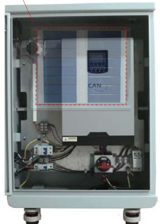
Battery pack behind the mounting panel
