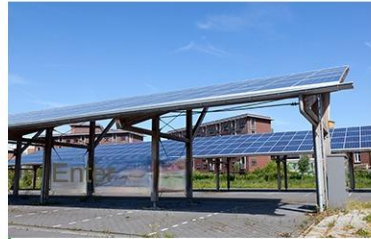
Parking Space Electricity
