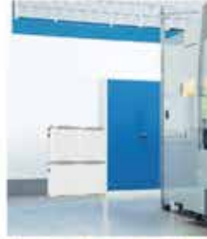
20kWh Shandong, China
