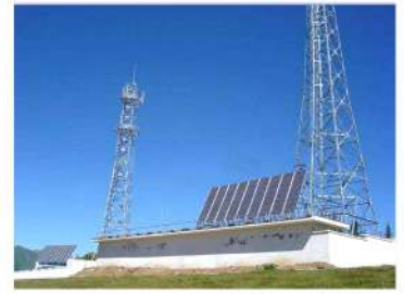
Communication base station, etc.
