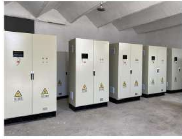
Energy storage system
