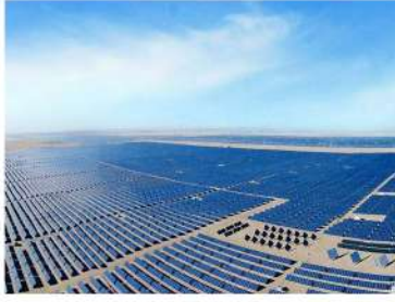
Photovoltaic power station
