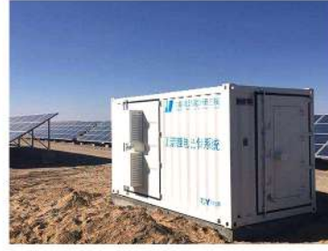
Photovoltaic energy storage system
