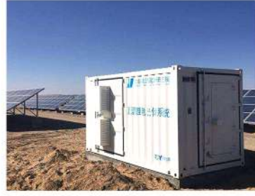
Photovoltaic energy storage system
