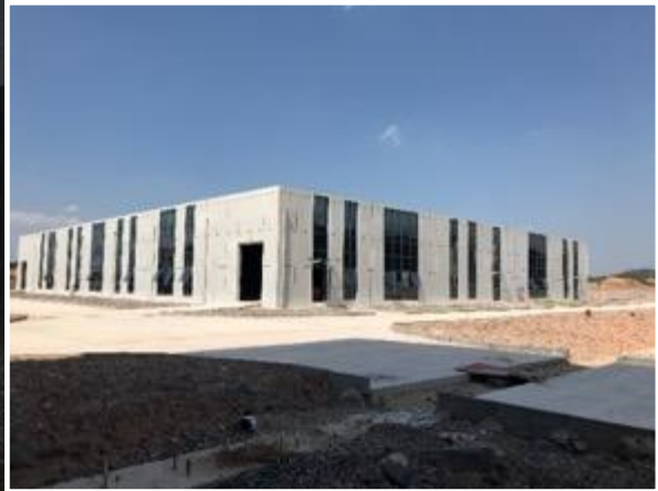
Battery Pack Assembling Line Building
