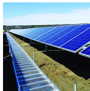
2 MW - Saratoga Springs New York
