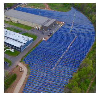
3.1 MW - Bridgewater New Jersey
