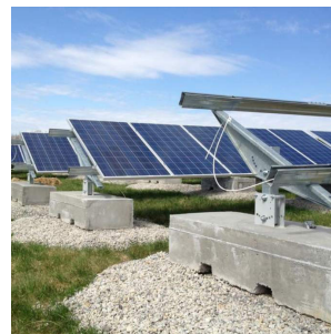
2 MW - Maynard Landfill Massachusetts
