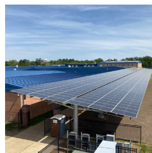
560 kW - Somerdale New Jersey
