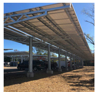
600 kW - Vineland New Jersey
