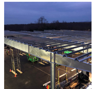
1.2 MW - East Windsor Connecticut
