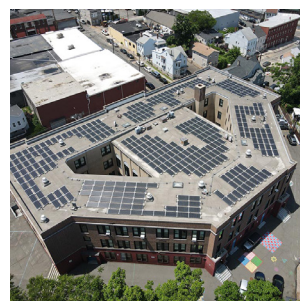
320 kW Patterson New Jersey
