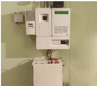
10KWh Puerto Rico
