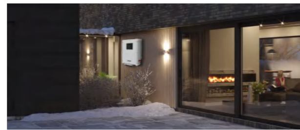
Residential Project in Poland 10kW
