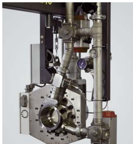
Process water piping
